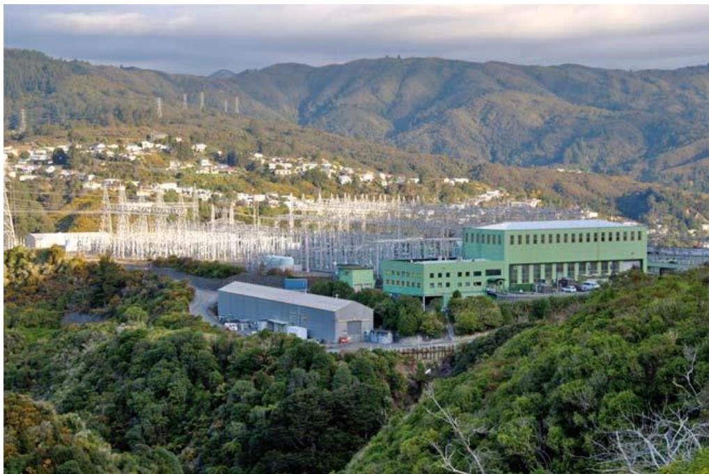
Figure 3-9 Haywards Converter station New Zealand
