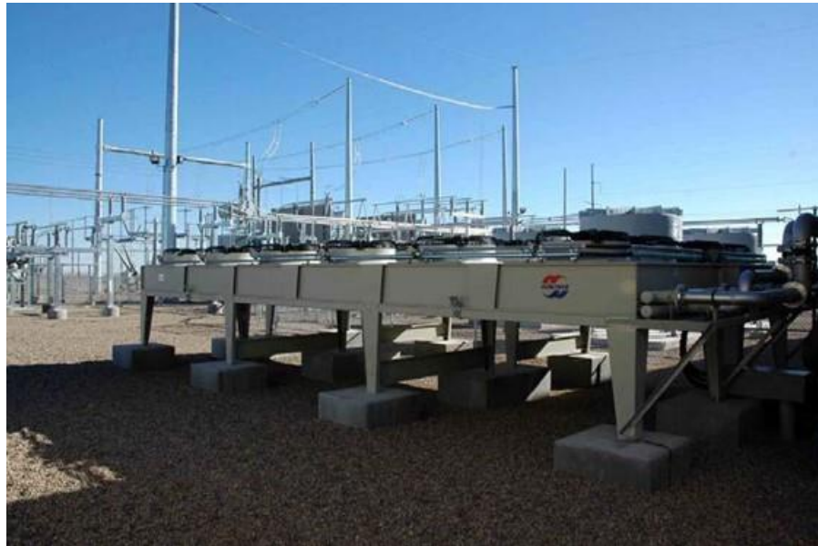
Figure 3-5 Outdoor Valve Cooling radiators and cooling fans
