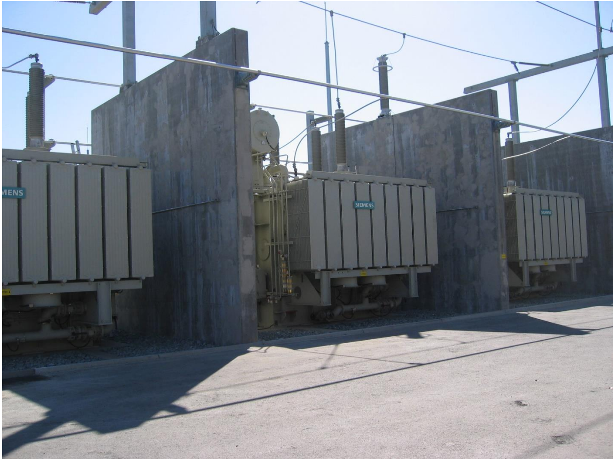
Figure 3-6 transformers with containment pits and barriers
