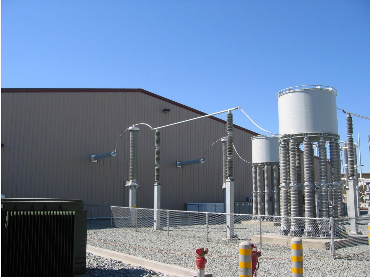
Figure 3-7 Air Core Dry Type Smoothing Reactor
