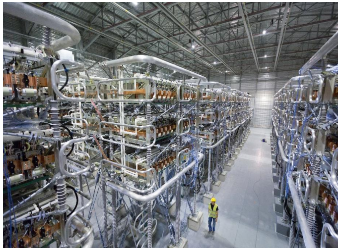
Figure 3-3 VSC converter valves courtesy of Siemens
